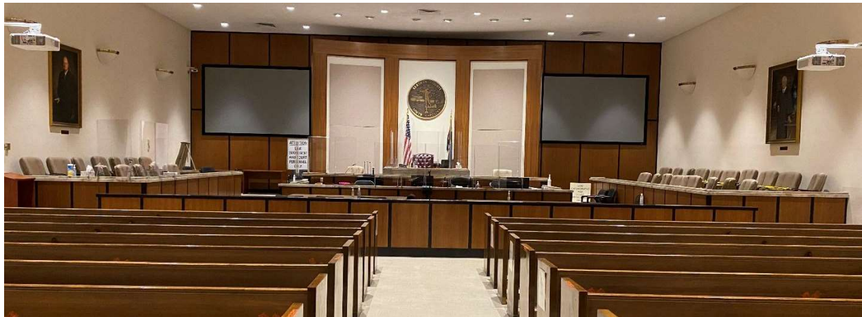
Circuit Court Room – new audio and video system
